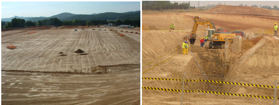
Fig. 2 ( left ) Overall view of the site as in August 3 rd 2006. ( right ) Digging the service gallery (September 2006).
